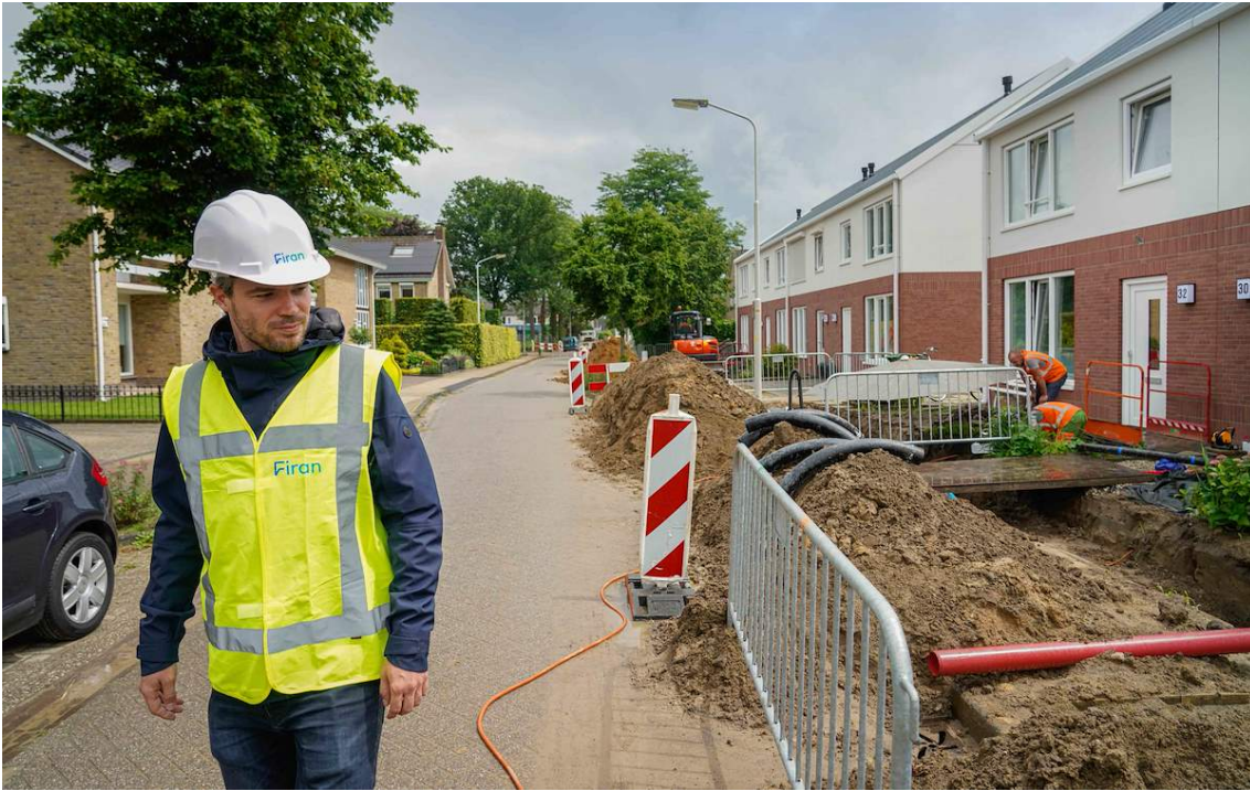
In 2024, we worked on developing and expanding district heating networks in various municipalities through our subsidiary Firan.
